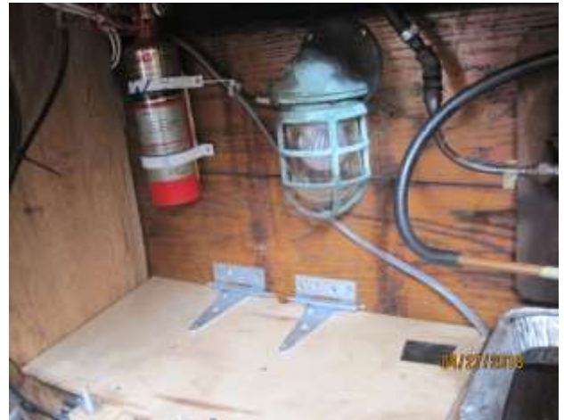
Fire Suppression System
